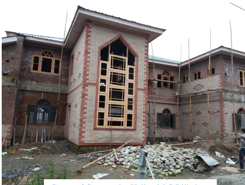
Const. of Community Hall at M.C Bijbehara Project Cost = Rs 202.14 lacs Expdt. 3/2016 = Rs 88.95 lacs
